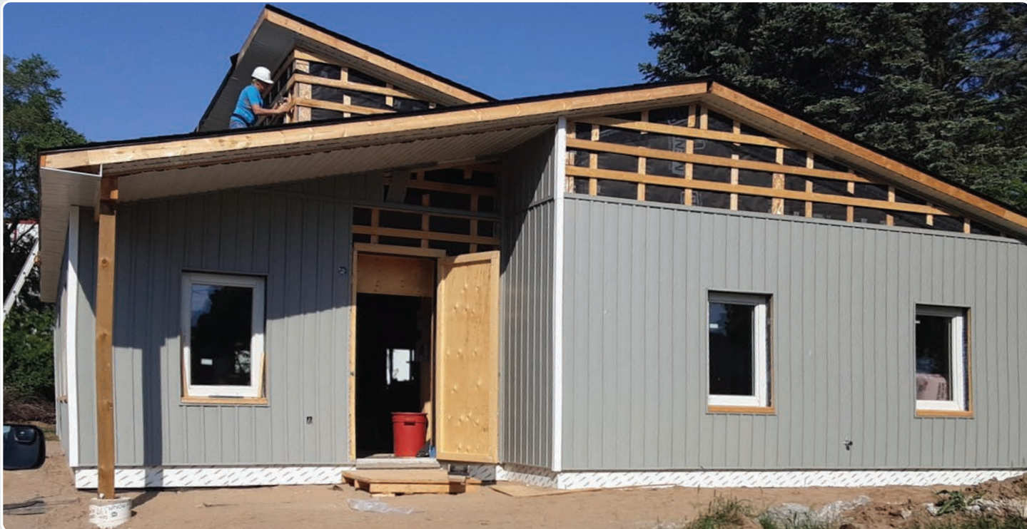
28 Willowdale St., Brant County, ON - Single family home built to passive* standards.
